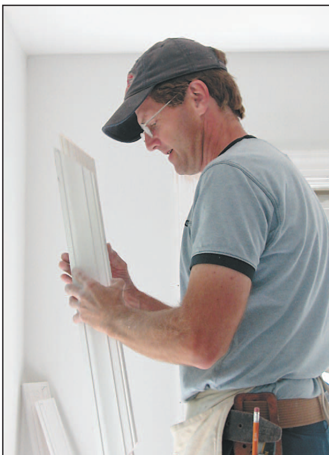
Danny Strunk of Cronshaw Carpentry sizes window casings to go into the first floor of the home in Oxford the company is remodeling.
